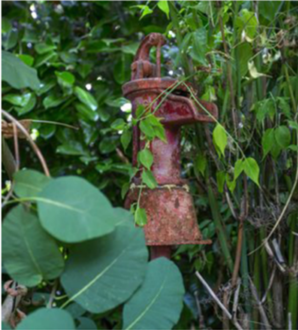
A rusty water pump is one of the many details that emphasize the age of the... (Mike Siegel/The Seattle Times)
